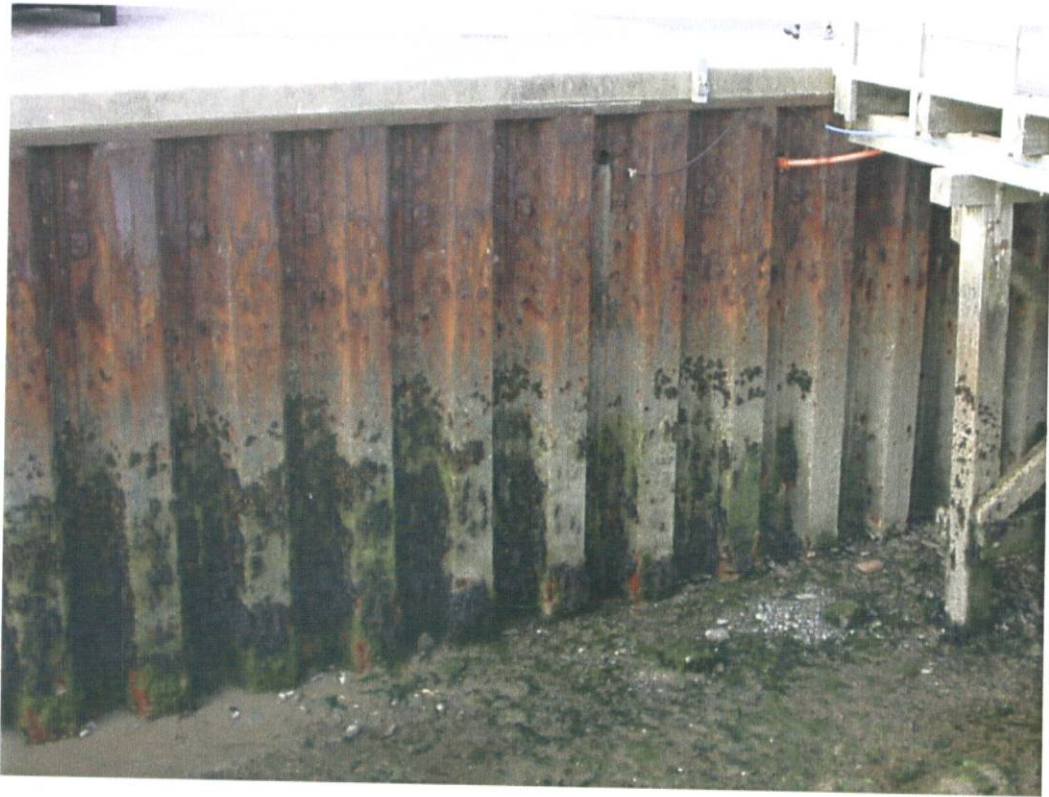
August 2003, note bright orange deposits at bottom of piling.
