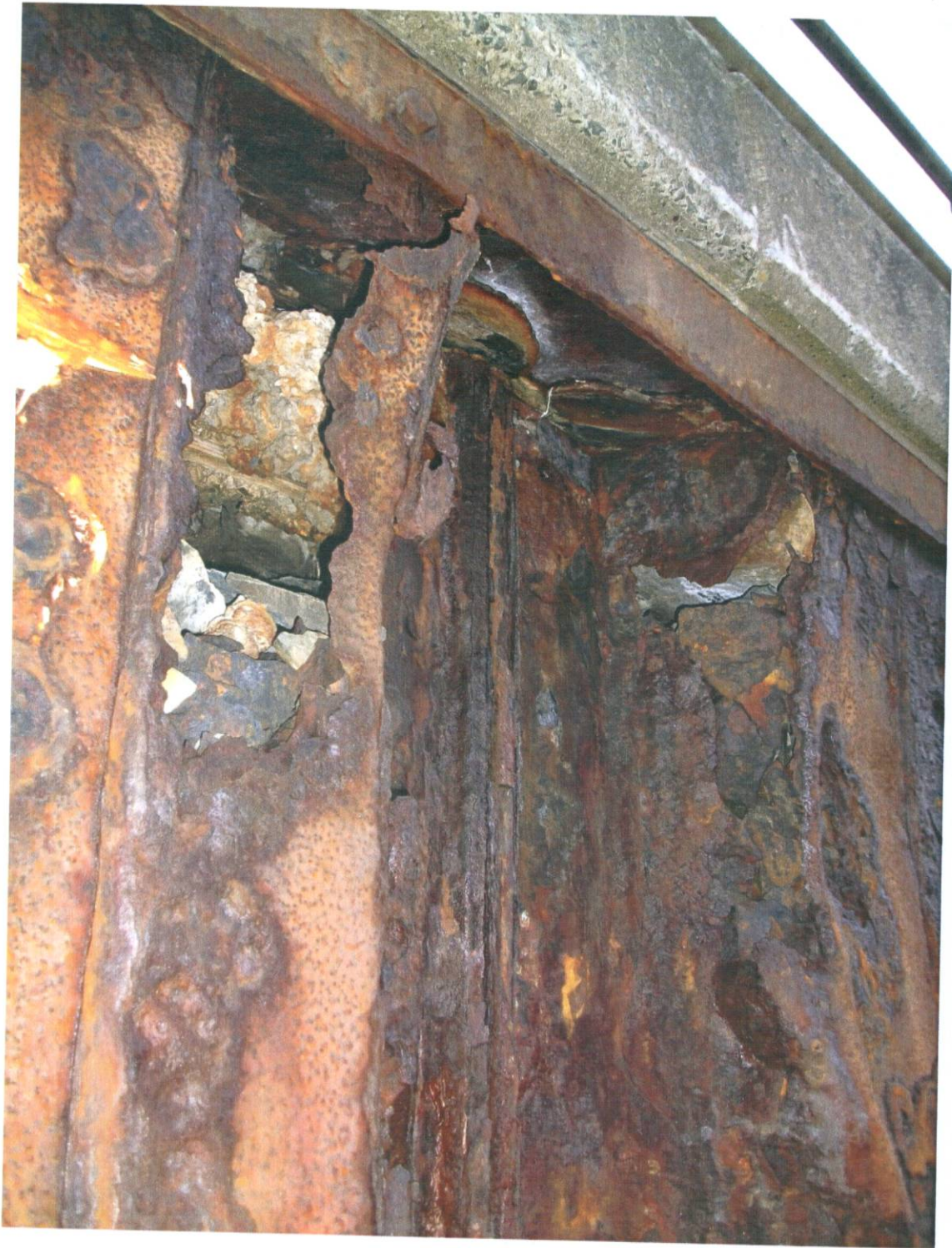
Impact damage to top of wharf wall.
